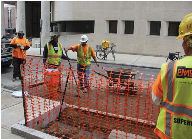
Workers from Emerge Connecticut Inc. construct a bioswale near the intersection of Wall and Church streets in New Haven in October.
