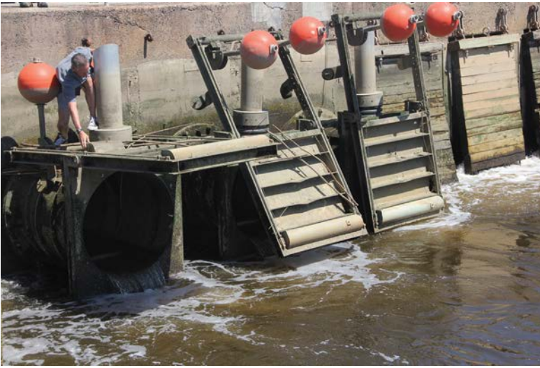
The self-regulating tide gates installed on the West River five years ago allow salt water to flow upstream, restoring a tidal marsh and reducing flooding in the surrounding area.
